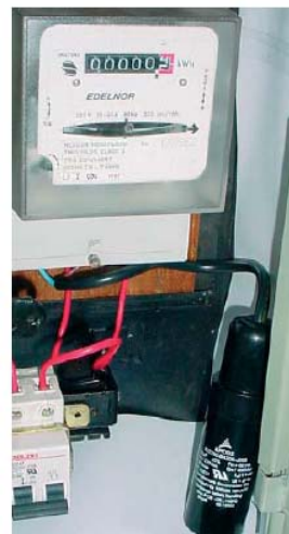
Fig. 6: HomeCap installation in the metering cabinet
